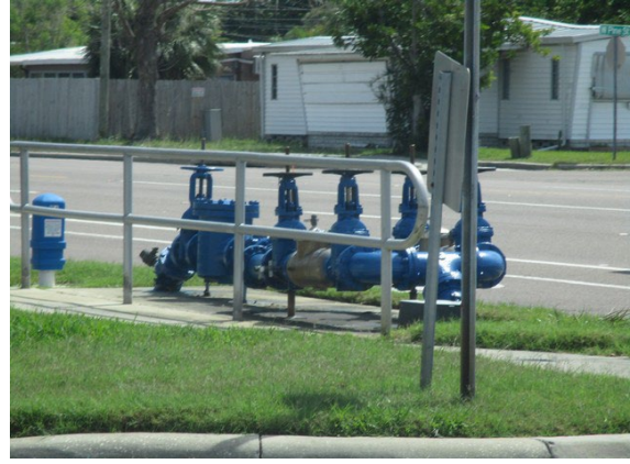
66 Main Valves/Backflow Preventer
