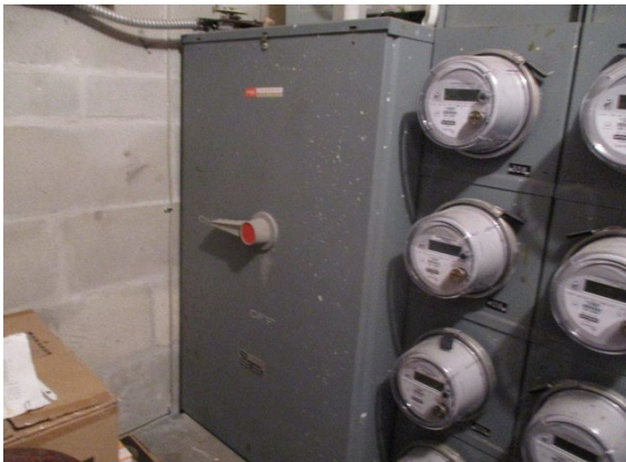
15 Meters & Main Panel
