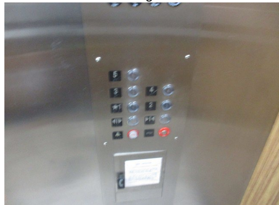
6 Elevator Cab Control Panel
