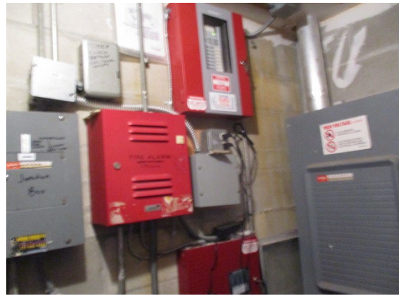
18 Fire Control Panel
