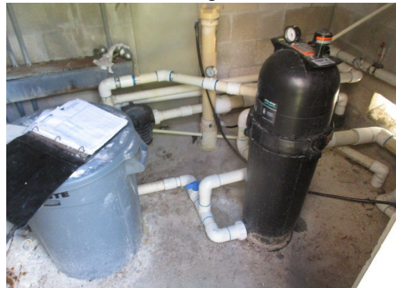
64 Pool Equipment (Shared)
