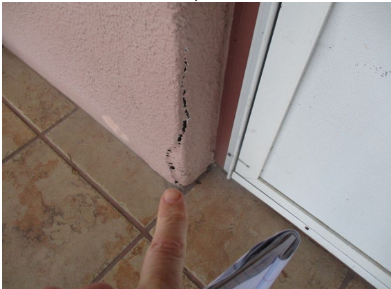
45 1st Floor Vertical Crack @ Unit #108 Doorway
