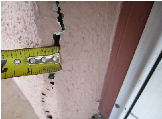
47 1st Floor Vertical Crack @ Unit #108 Doorway
