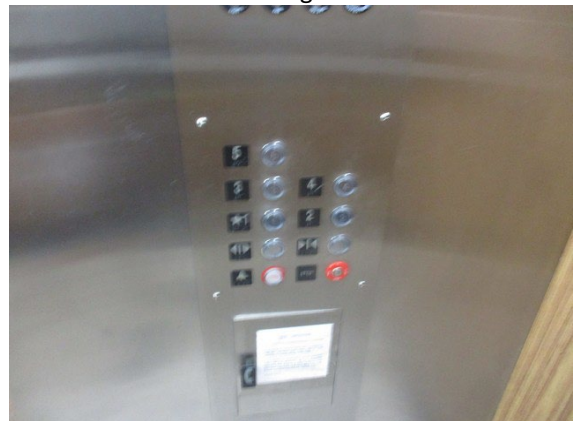
6 Elevator Cab Control Panel
