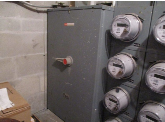
15 Meters & Main Panel
