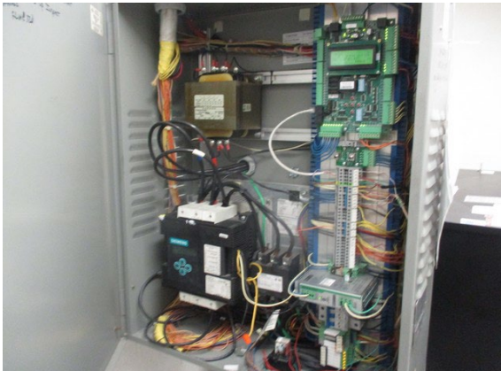
29 Elevator Control Board
