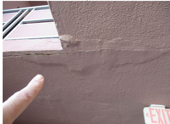
38 3rd Floor Walkway Ceiling Stucco Bulging At Expansion Joint
