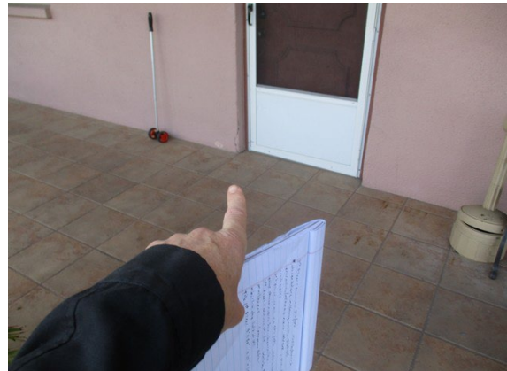
46 1st Floor Vertical Crack @ Unit #108 Doorway
